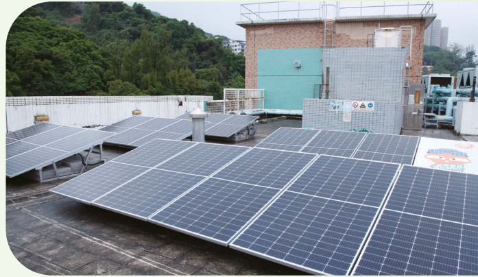
靈實在院舍安裝太陽能發電板。 Solar panels have been installed in our residential care homes.
